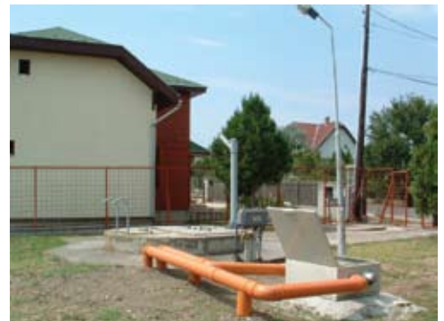
Biothys BAF deodorising system (sewage water treatment)
